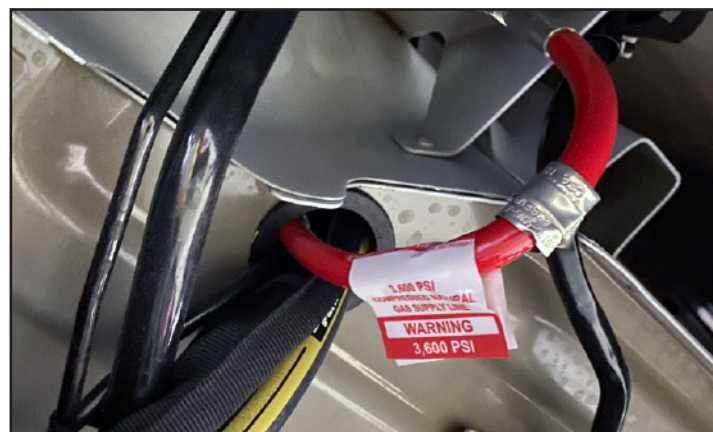
All high pressure hoses must be labeled with a high pressure sticker.
